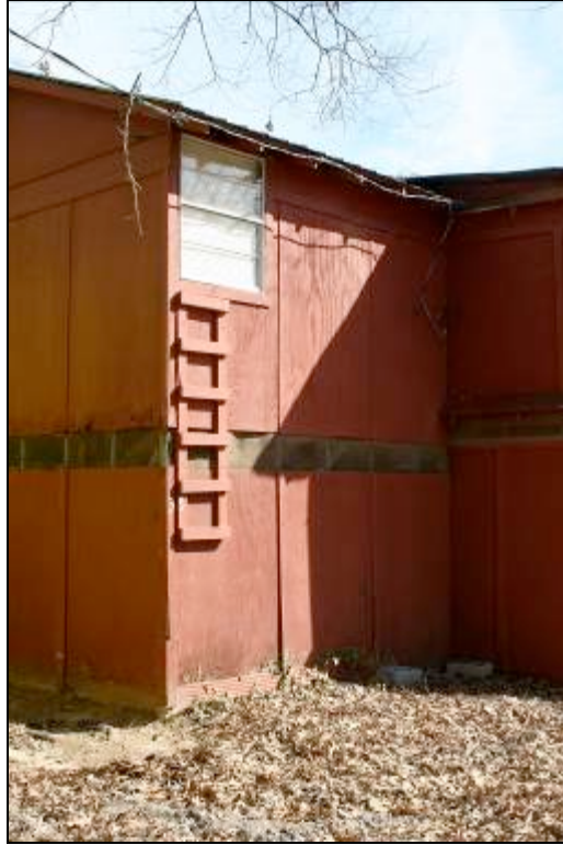
Figure 2.13 An example of how cabin owners vent the heat from the cabins.
